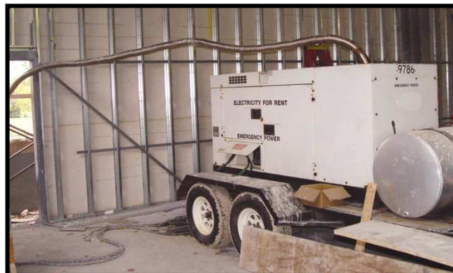
Good example of generator exhausts being vented to the outside.
