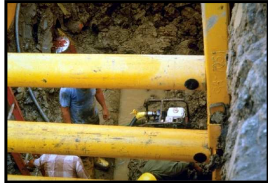
Gasoline engine (water pump) being operated inside a trench box (enclosed space); this is a potential hazardous exposure to carbon monoxide!
